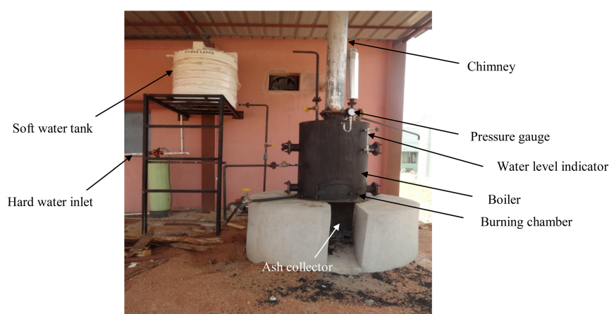
Fig. 2. Set up of Steam boiler and softener.
